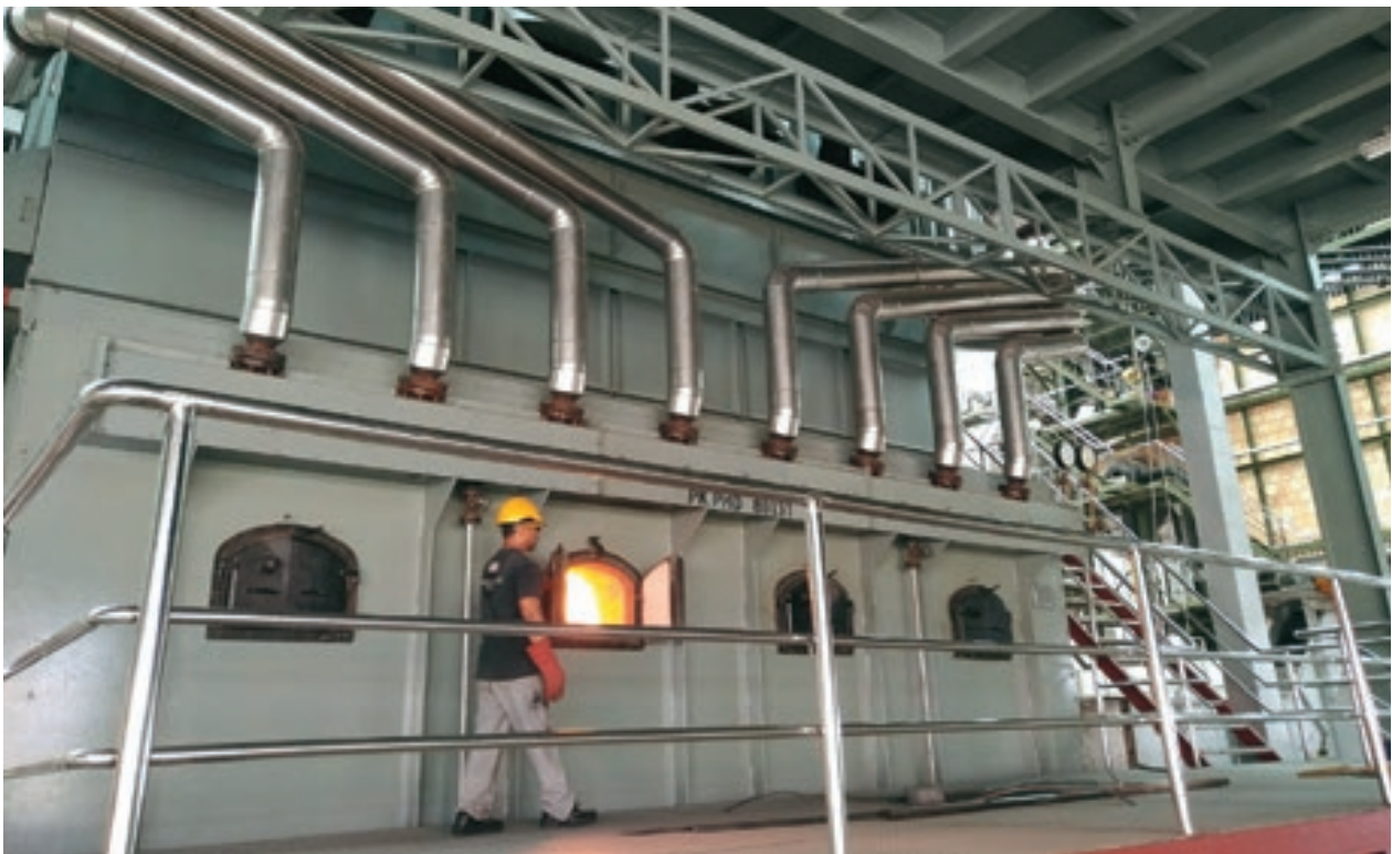
The new biomass Reciprocating Boiler at the Optimill commissioned in November 2017.
