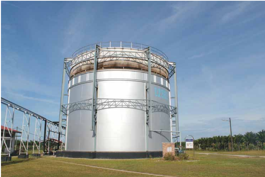
The Jendarata Estate Biogas Plant commissioned in 2006 treating the Palm Oil Mill Effluent. In the process of reducing the Biochemical Oxygen Demand by 99%, biogas is produced by methane bacteria and subsequently used as a source of green energy.
