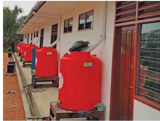
Water tanks are supplied for harvesting rain water.
