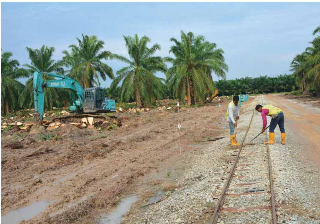
Railway tracks maintenance in progress next to a field that is being replanted.
