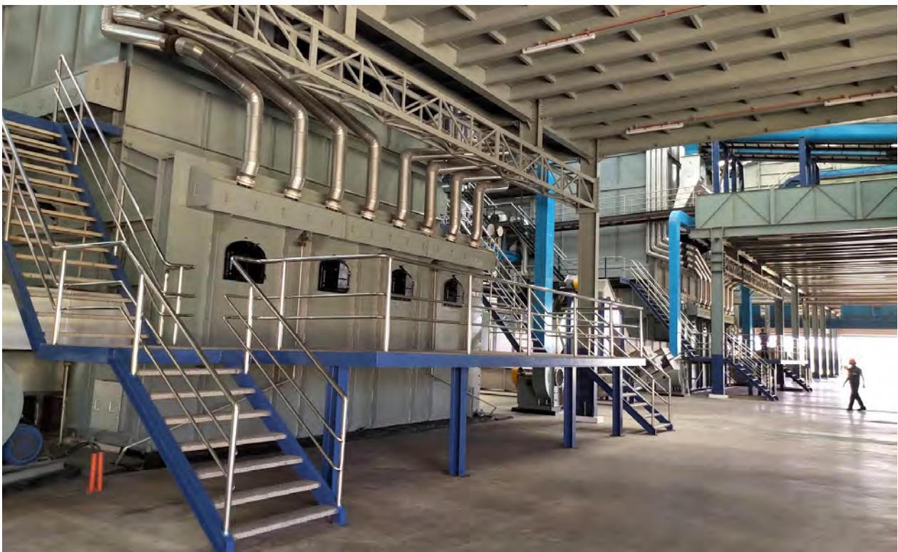
Biomass Reciprocating Boilers at the Optimill.
