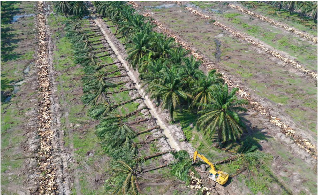
A vital part of sustaining soil health is to ensure that the large amount of biomass from the oil palm trunk and fronds is returned to the soil during replanting operations in line with our Zero Burn policy. More than 1,100 Ha of old standing palms have been felled since UP took over Pinehill estate (Tanarata) on the 17 August 2019.
