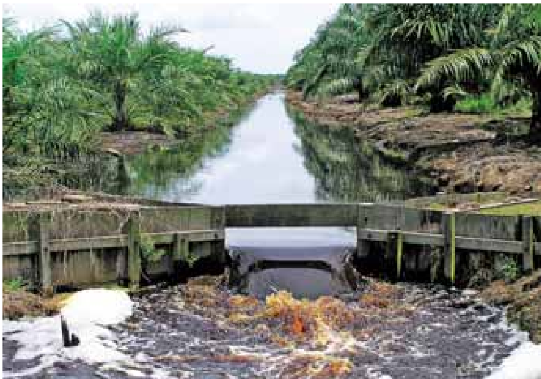
Wooden weirs are important tools to regulate the height of the water tables in the fields.
