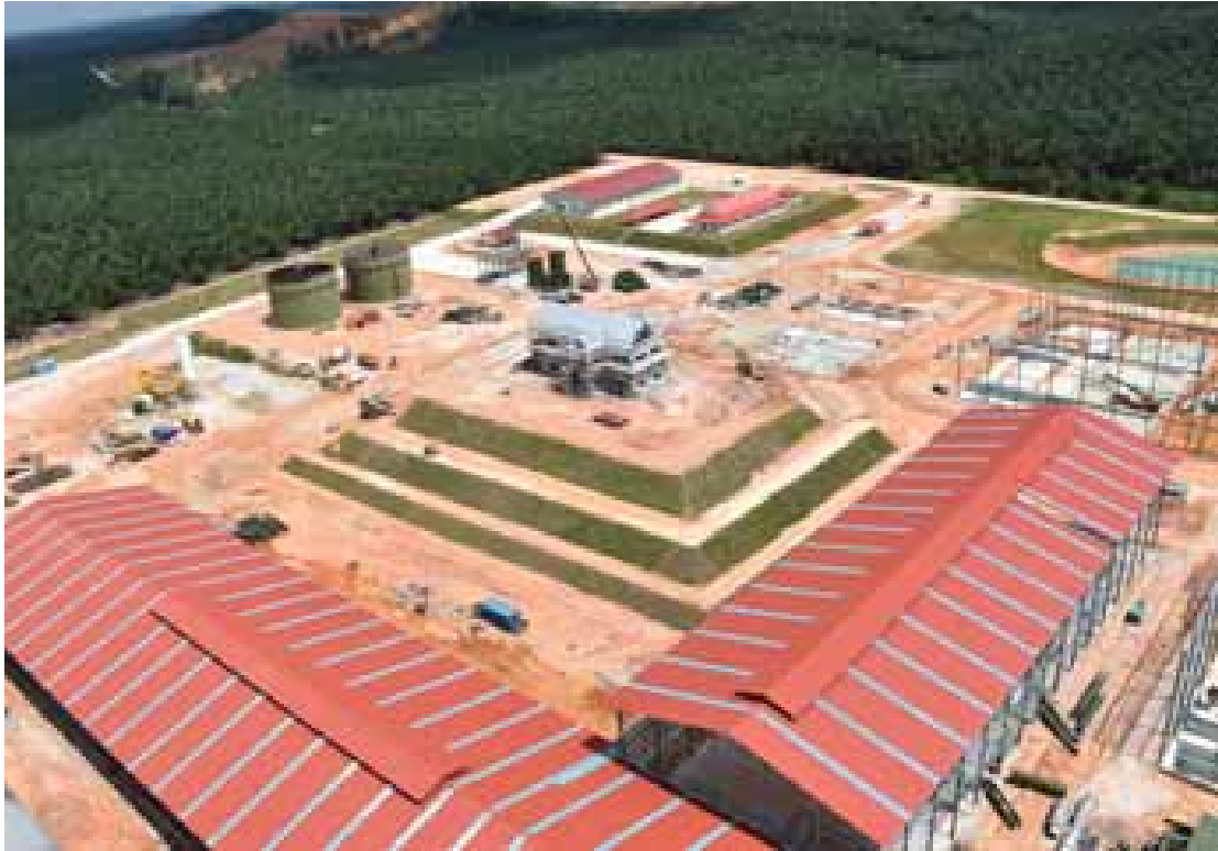
The construction of the in-house designed 60 tonne per hour Optimill which upon commissioning will not only stand out aesthetically but just as importantly become an example of fulfilling the “circular economy”.
