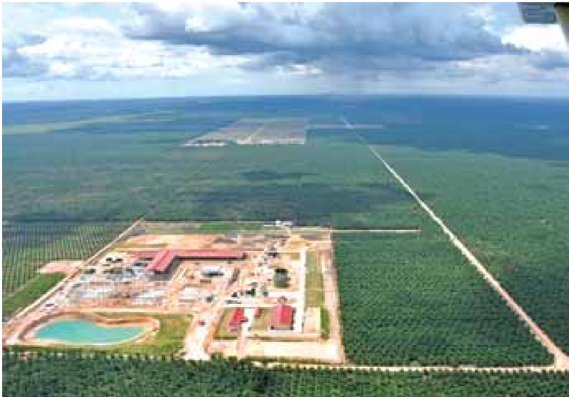
Aerial view of the construction progress made at the Optimill in Ulu Bernam.
