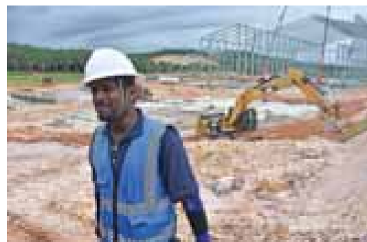
The safety superintendent, Mr. Kalai during his daily inspections at the Optimill construction site.
