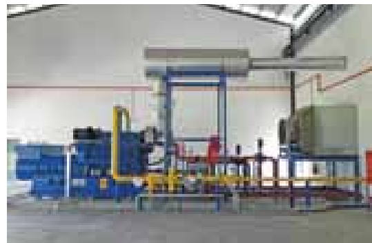
Newly installed Biogas Engine for electricity generation.
