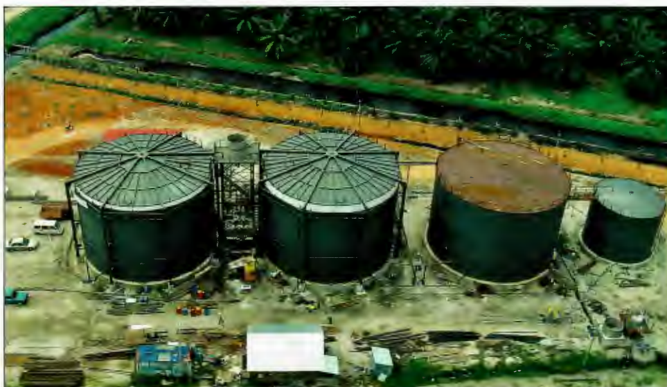
An aerial view of the Biogas Plant at Jendarata Estate commissioned in commemoration of the company's 100 years of operation in Malaysia. (September 2006)
