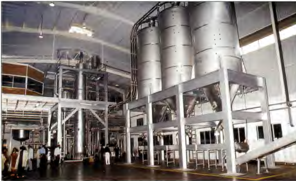
The fully continuous Saponification Plant which was commissioned at Unitata Berhad in 2004, enabling the Company to expand its range of high quality toilet soap noodles and specialized finished products.
