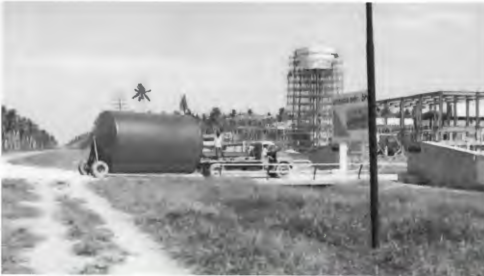
Unitata Berhad, the first inland palm oil refinery in Malaysia under construction during the early 1970's. It was commissioned in 1974.
